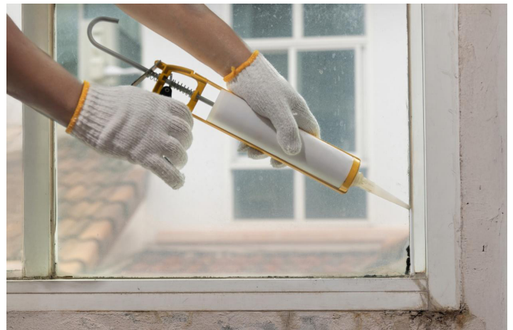
Sealing window gaps to stop air leaks and improve energy efficiency. Adobe Express photo
