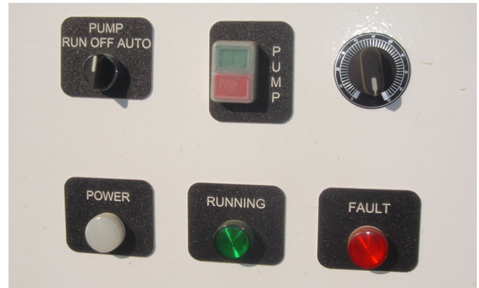
VFD pump panel controls. Auto (sensor driven) or manual mode (upper left), start/stop (top center), variable speed dial (upper right), power to panel indication (lower left), VFD operational indication (bottom middle) and fault indication (lower right).
