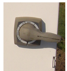
Safety shutoff/lockout for VFD panel.
