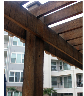
This pergola's beams have been affixed to the sides of the vertical posts.
