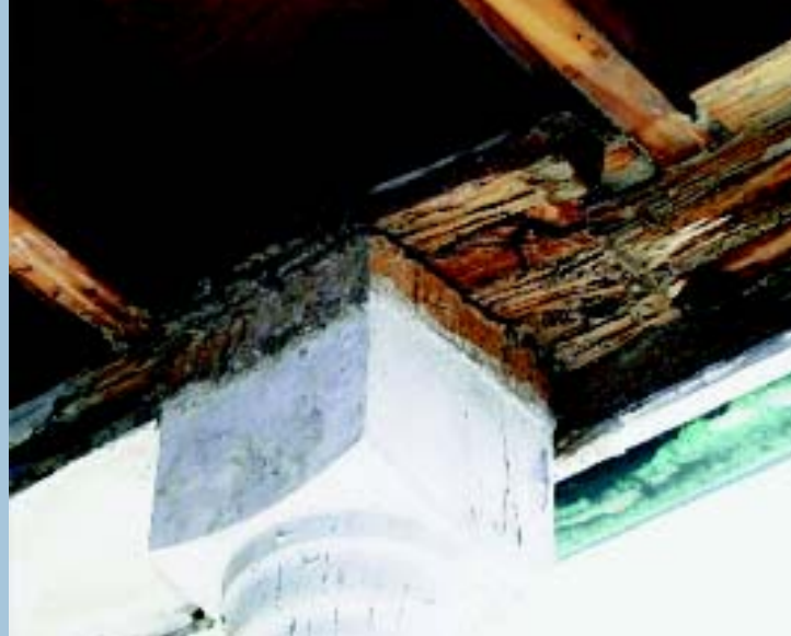
Photo 24. Wood above pillar damaged by Formosan subterranean termite
