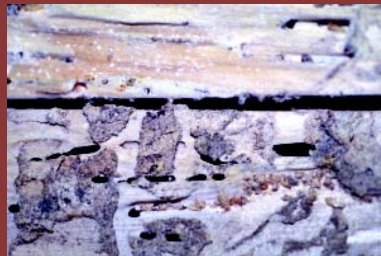
Photo 11. Wood damaged by subterranean termite: galleries with soil
