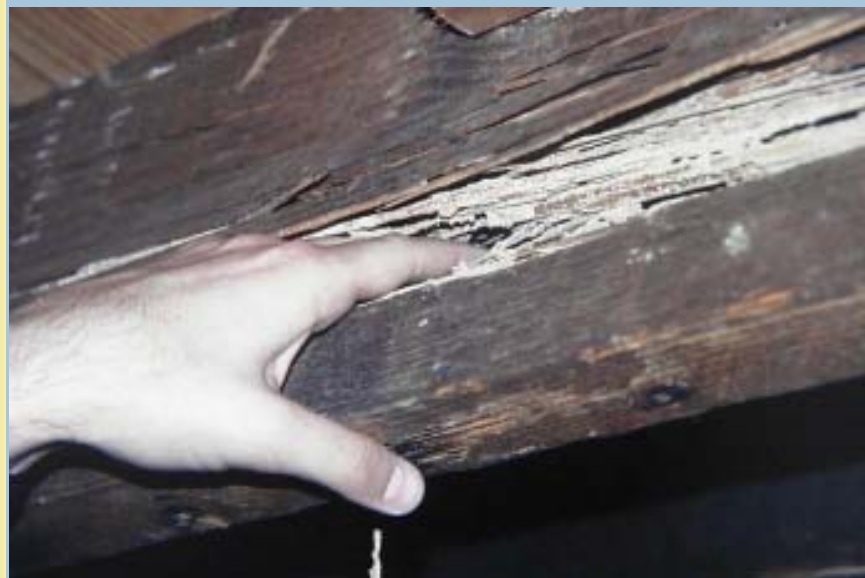
Photo 25. Beam damaged by Formosan subterranean termite
