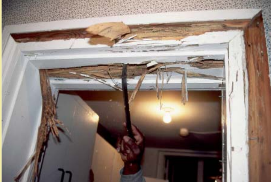
Photo 23. Wooden door frame damaged by Formosan subterranean termite
