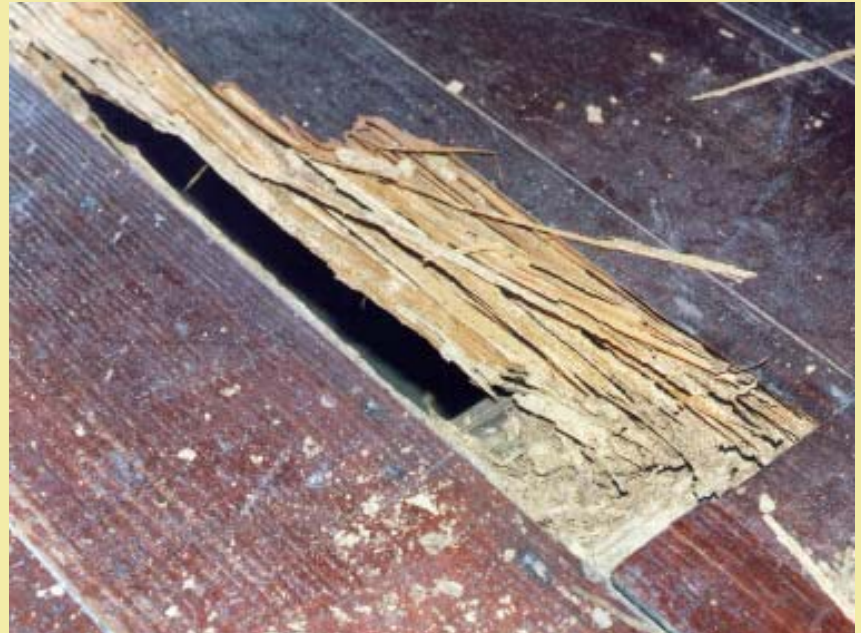
Photo 22. Wooden floor infested by Formosan subterranean termite
