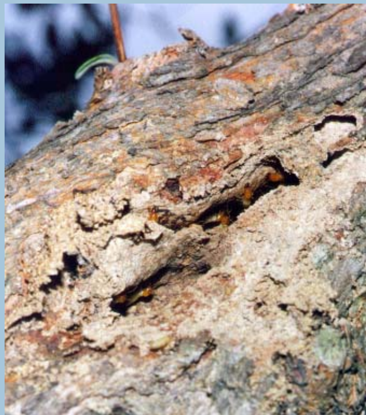
Photo 26. Living tree infested by Formosan subterranean termite
