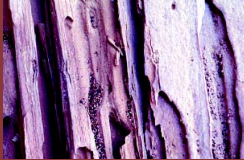
Photo 7. Wood damaged by drywood termite: large and smooth galleries across and with the grain, with dry and six-sided fecal pellets
