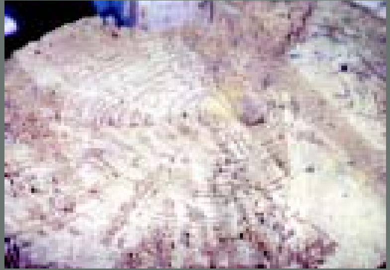
Photo 13. Wood damaged by subterranean termite: showing damage along grain
