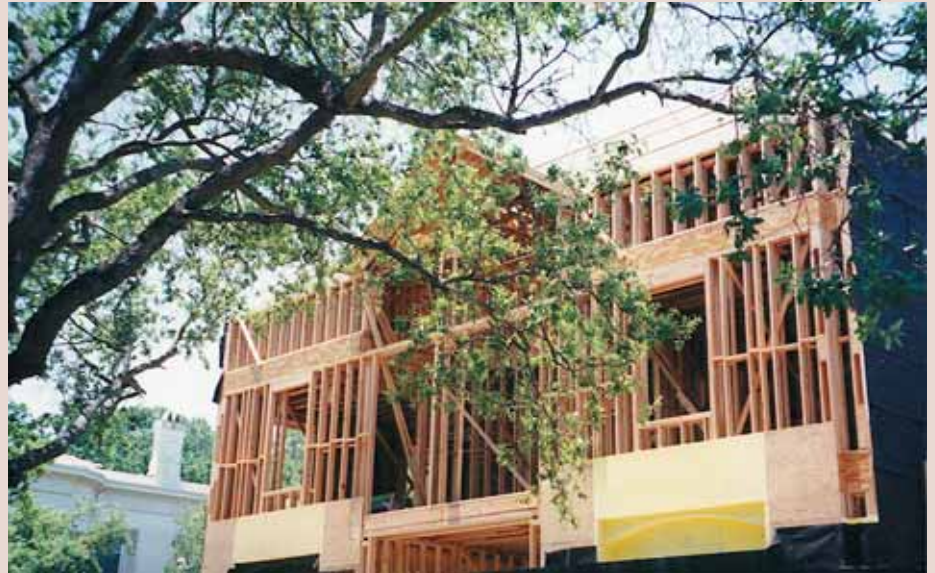
The Louisiana Forest Products Laboratory is testing wood treatments that will protect structural materials from termites. This house in New Orleans is being constructed with borate-treated lumber. Borates have been found to be toxic to termites.
