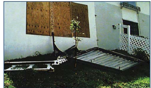
Figure 3 Hurricane Georges in Puerto Rico. The window lying on the ground was protected by a shutter. However, the shutter was attached to the window frame. The window frame fasteners were over-stressed and the entire assembly failed. Attachment of the shutter directly to the wall framing is a more reliable method of attachment.
