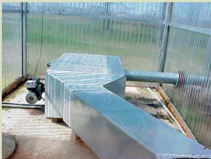
Figure 2. One modification is to use a floor heater connected to an 18-inch duct for heat transfer.
