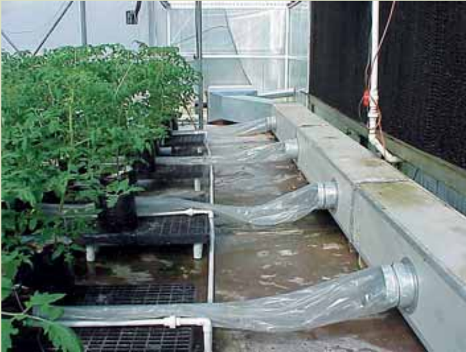
Figure 3. Warm air is piped through perforated poly tubes.
